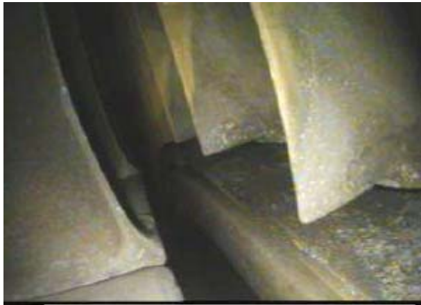
Minor Deposits on HPC blades/vanes
